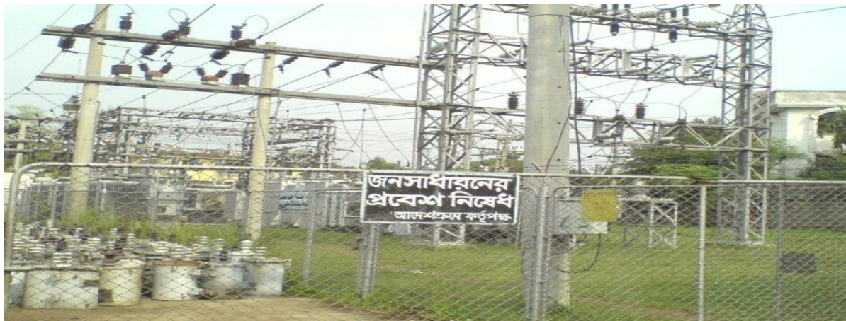
Figure 17: Overall View of the Distribution Substation (author)
