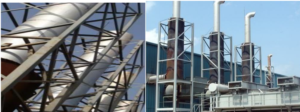
Figure 9: Radiator with 14 fans at UPGD [3]
