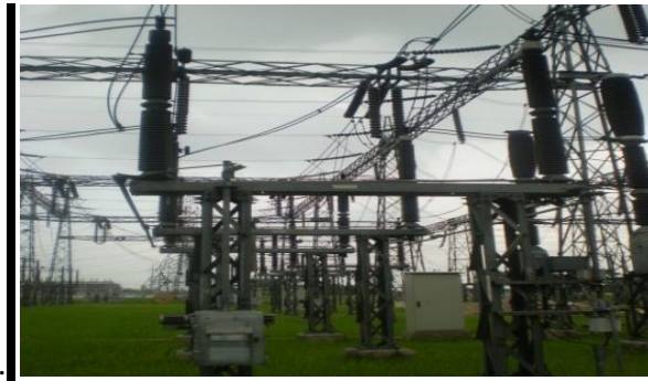
Figure 4.3: Part of a Substation of APSCL
