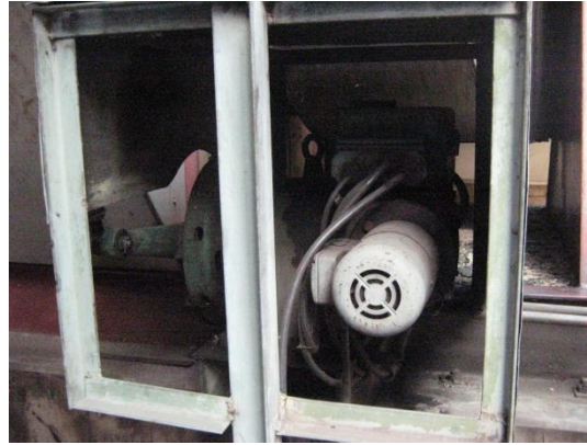
Figure 2.12: Forced Draught fan actuator unit-3
