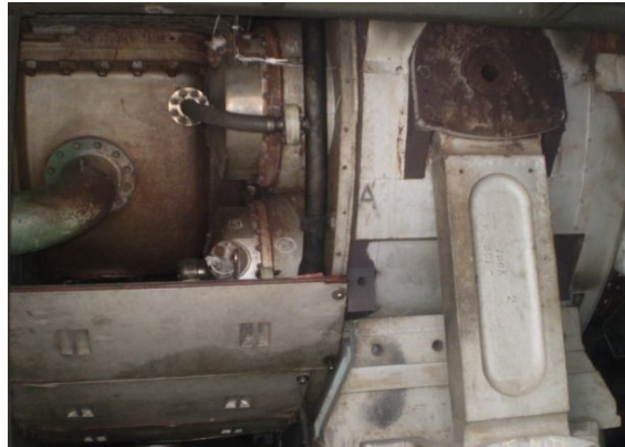
Figure 3.3: Combustion Chamber of Gas Turbine Plant of APSCL
