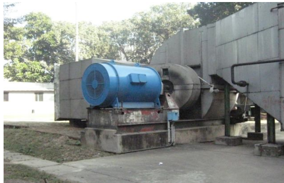
Figure 2.11: Force Draught Fan unit-3
