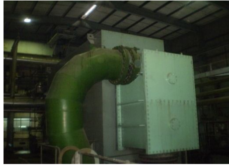
Figure 3.7: Condenser used in steam turbine section of combined cycle power plant (APSCL)
