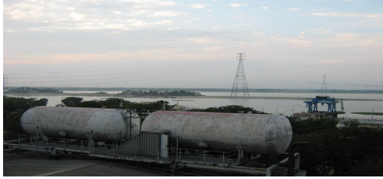
Figure 2.9: Feed Water Tank unit-3
