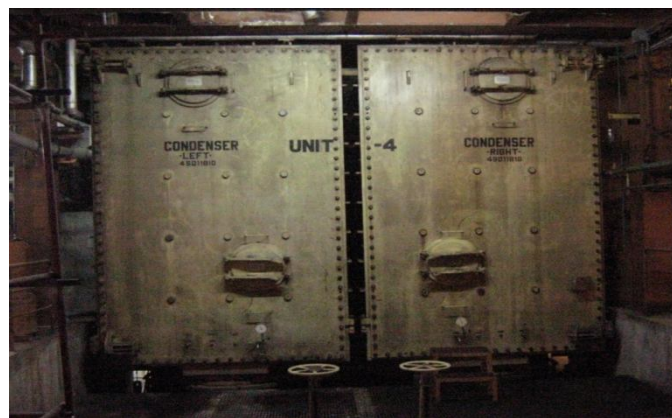
Figure 2.7: Condenser of unit -4
