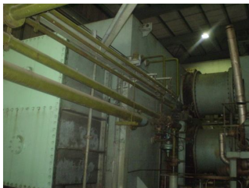
Figure 3.2: Centrifugal compressor used in APSCL
