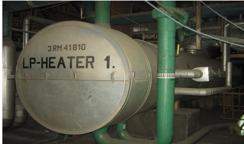
Figure 2.8: LP heater of unit-3
