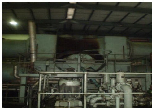
Figure 3.4: Gas turbine of APSCL
