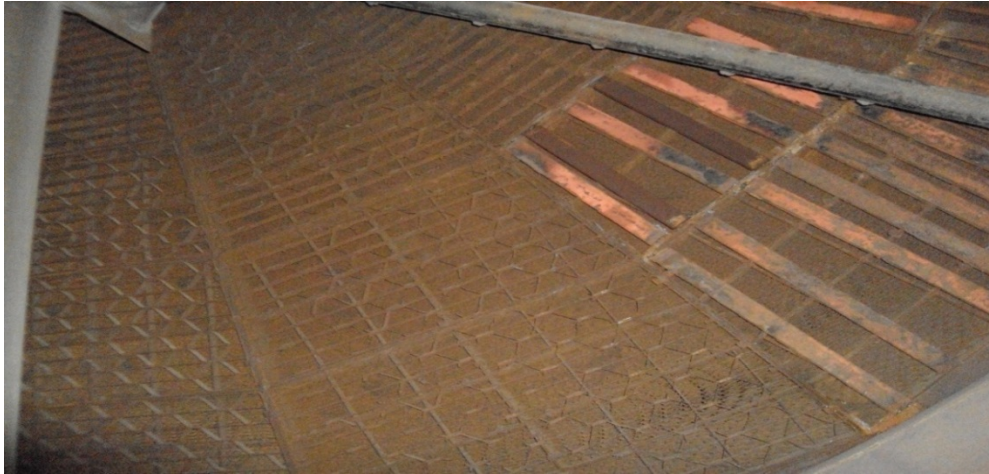
Figure 3.3: Inside view of air pre-heater in APSCCL.
