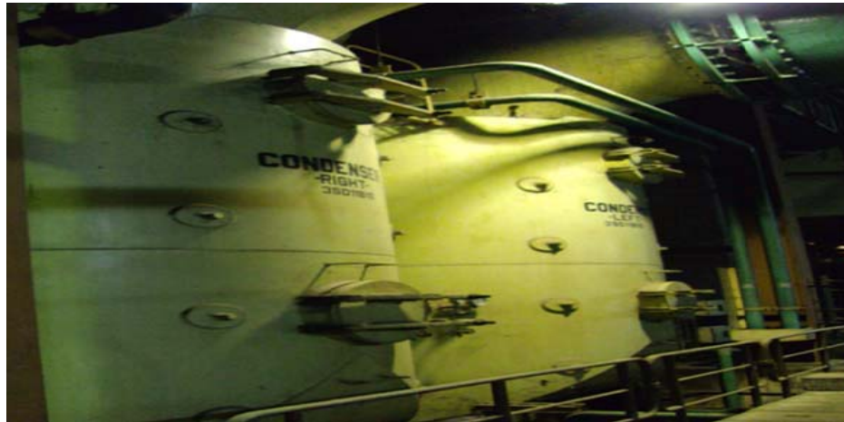
Figure 3.5: Condenser of steam power plant
