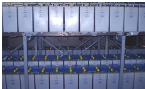
Figure 6.20: Battery room at APSCL substation
