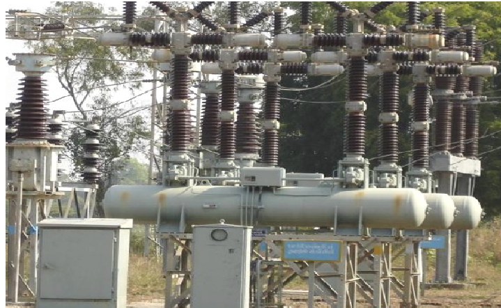
Figure 6.7: Air Blast Circuit Breaker used at APSCCL Substation
