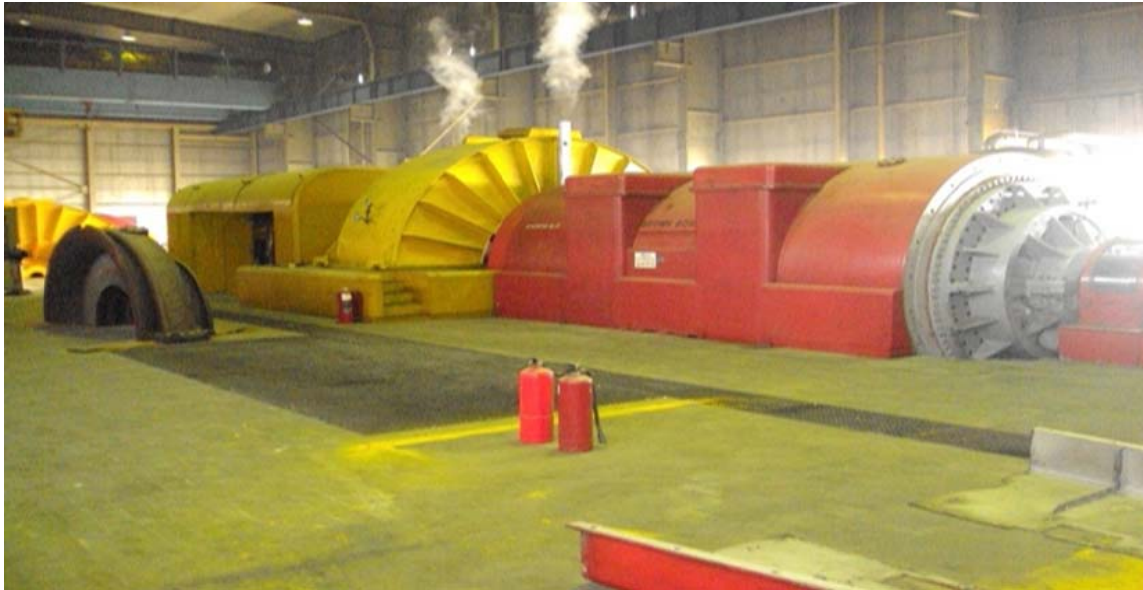
Figure 2.1: Generator of APSCL
