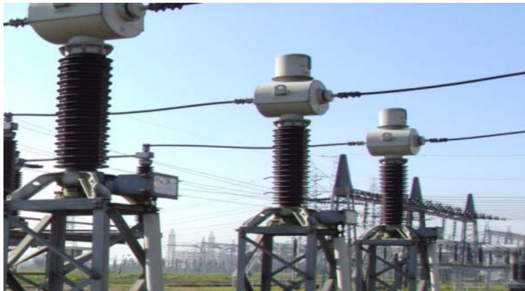
Figure 6.3: Current Transformer used at APSCL Substation
