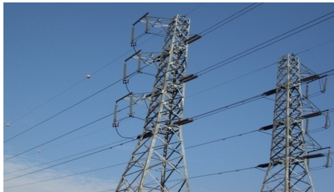
Figure 6.21: Overhead line of APSCL
