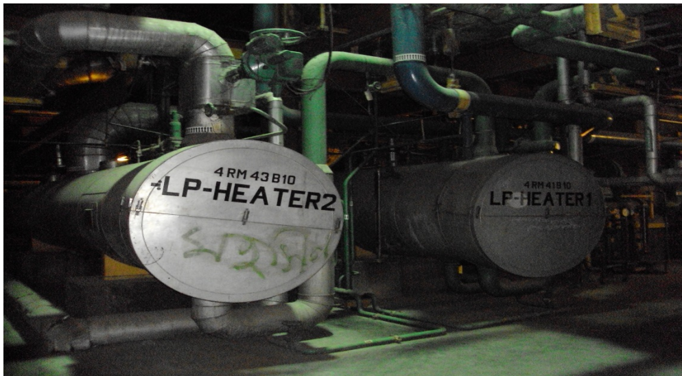
Figure 3.7: LP heater of steam power plant of APSCL
