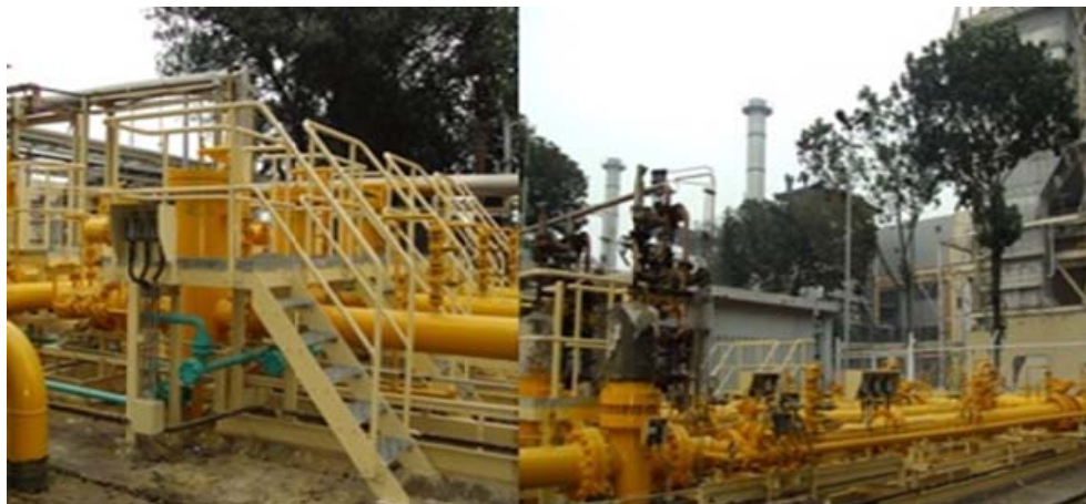
Figure 3.8: Gas pressure reducing plant.
