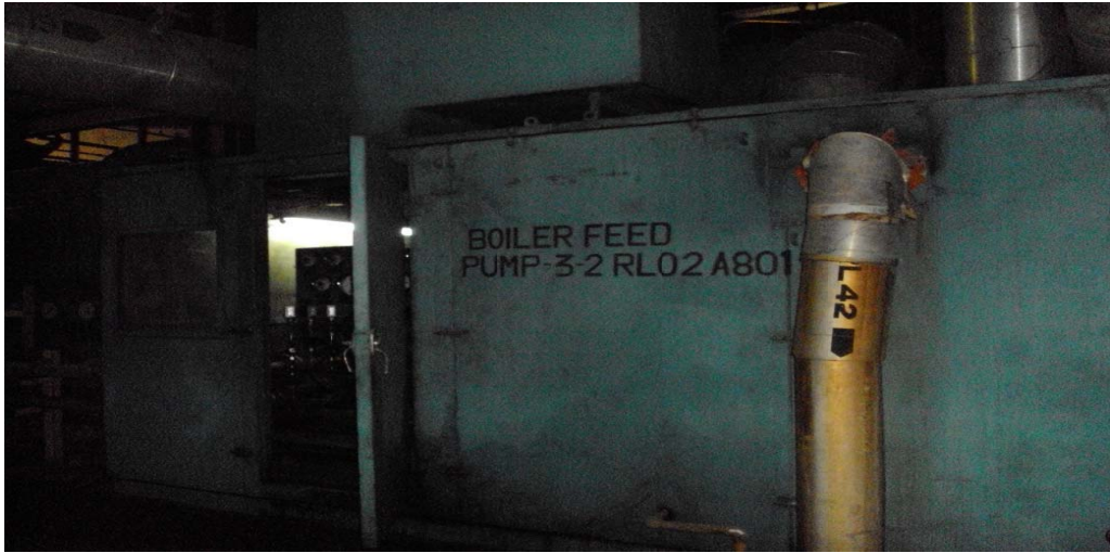
Figure 3.9: Boiler feed pump of APSCL
