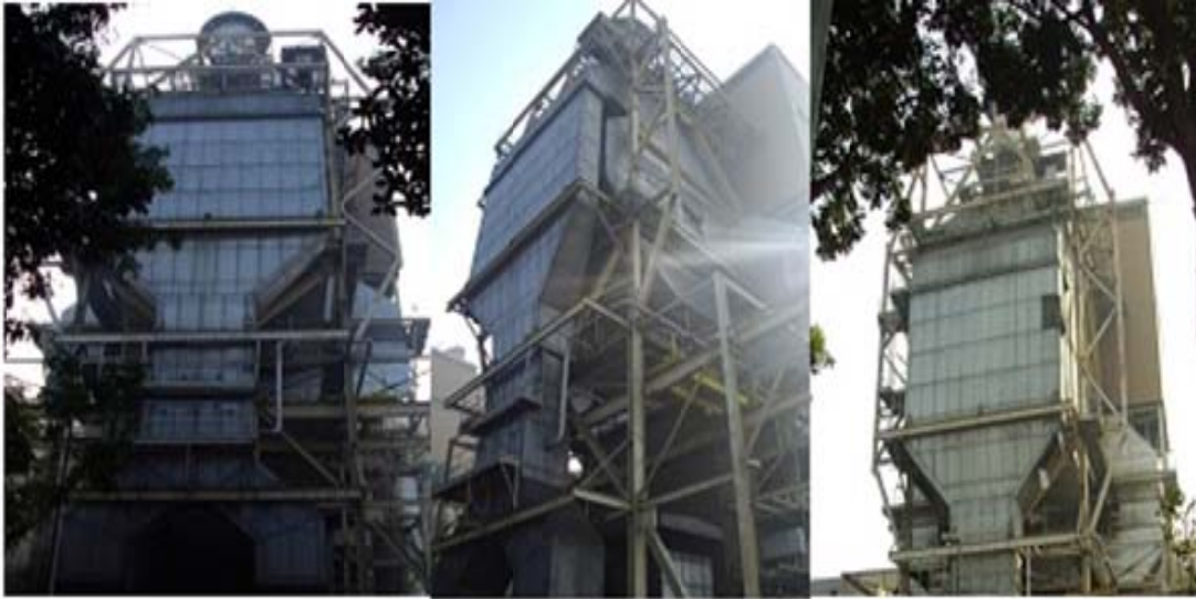
Figure 3.2: Boiler in APSCL
