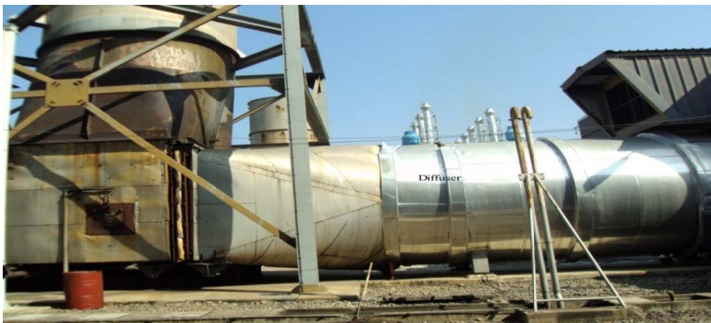
Figure 4.9: Diffuser in APSCL
