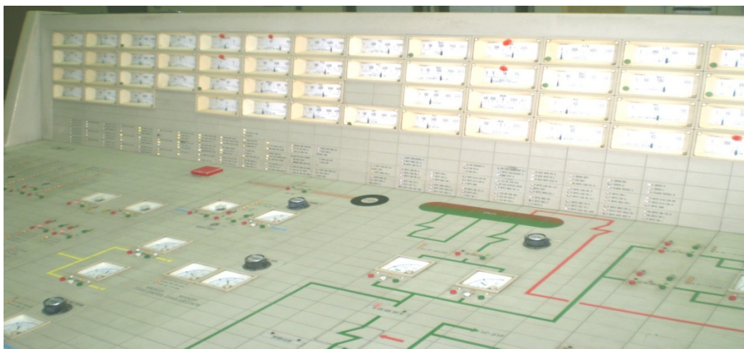
Figure 5.1: Control room of unit-5
