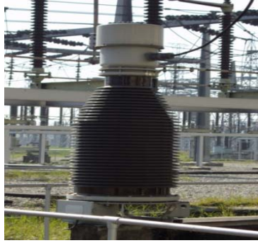
Figure 6.4: Potential Transformer used at APSCL Substation (132 kV single phase outdoor types)
