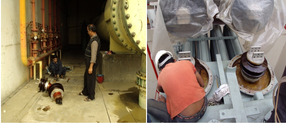
Figure 6.2 : Bushing is connected for power transformer at APSCL Substation
