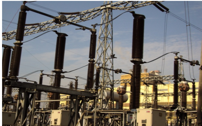
Figure 6.6: Oil Circuit Breaker used at APSCL Substation
