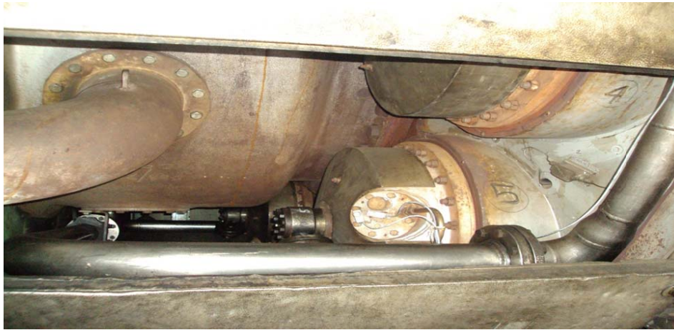
Figure 4.8: Inside view of combustion chamber in CCPP
