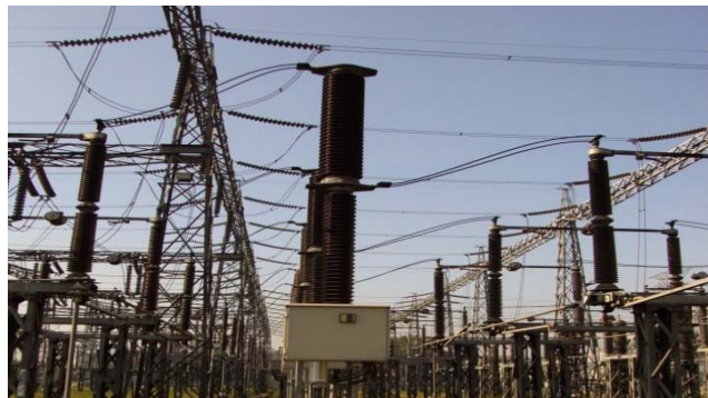
Figure 6.15: Double Bus-bar Connection used at APSCL Substation
