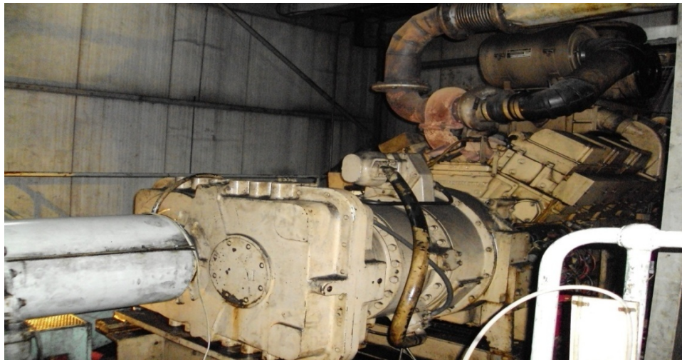
Figure 4.6: Diesel engine of combined cycle power plant
