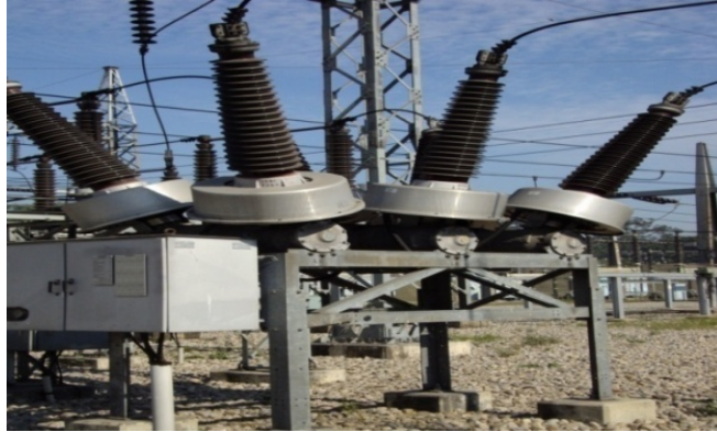
Figure 6.5: SF 6 Circuit Breaker used at APSCL Substation
