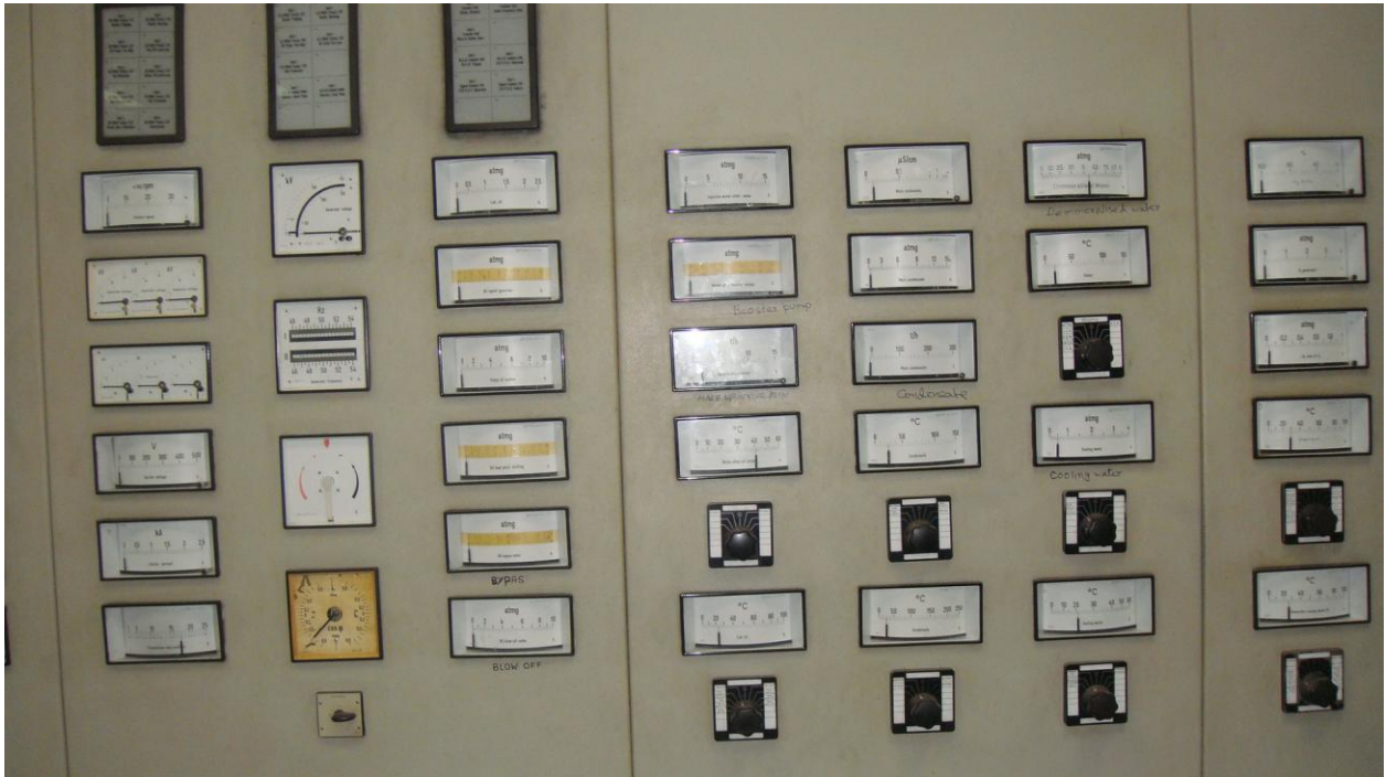
Figure 6.2 Control Room of Unit 1 & 2. [Source: Author]
