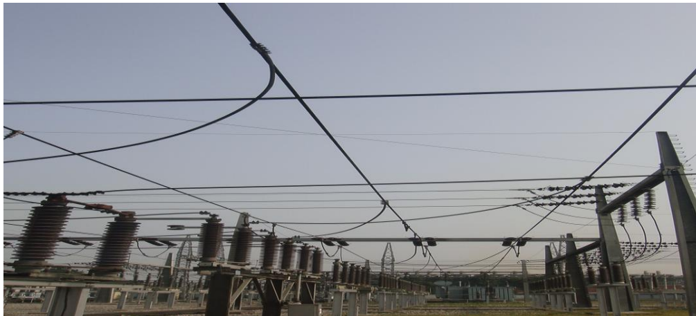
Figure 4.1: A typical bus bar of a substation [Source: Author]
