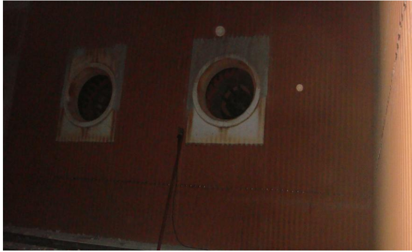
Figure 2.5: Burner room and water tube boiler. [Source: Author]
