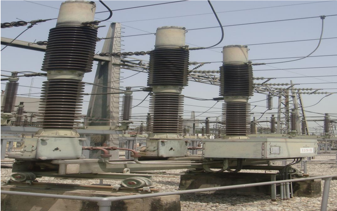
Figure 4. 21:Oil circuit breaker use in APSCL. [Source: Author]
