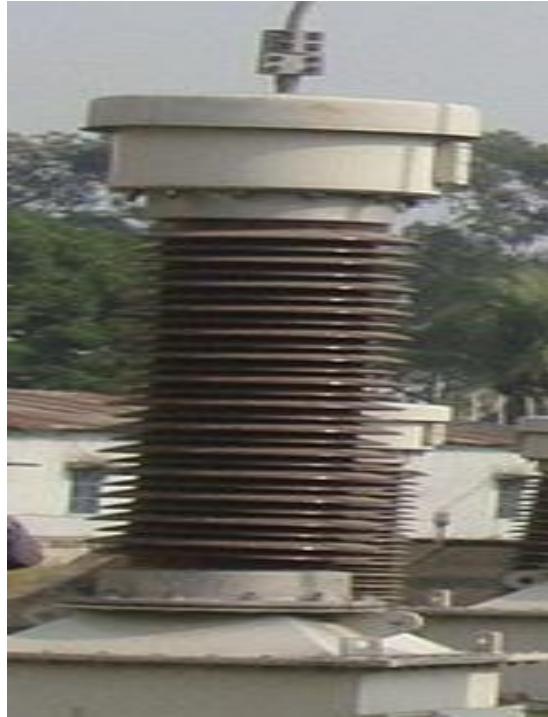
Figure 4. 3: A typical potential transformer (PT) [Source: Author]
