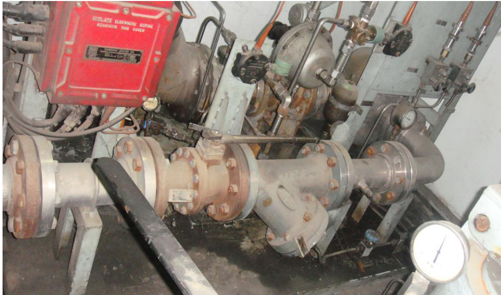
Figure 3.5 Fuel annex room in combine cycle power plant of APSCL.
