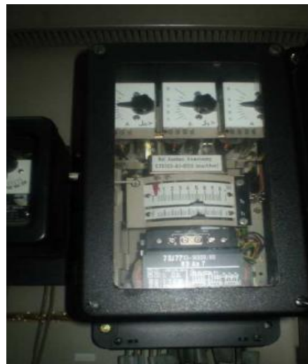
Figure 5.18: Picture of back up earth fault relay in APSCL. [Source: Author]
