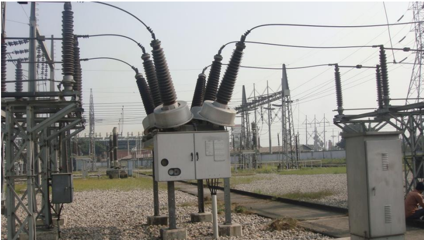
Figure 4.20: SF6 circuit breaker used in APSCL. [Source: Author]
