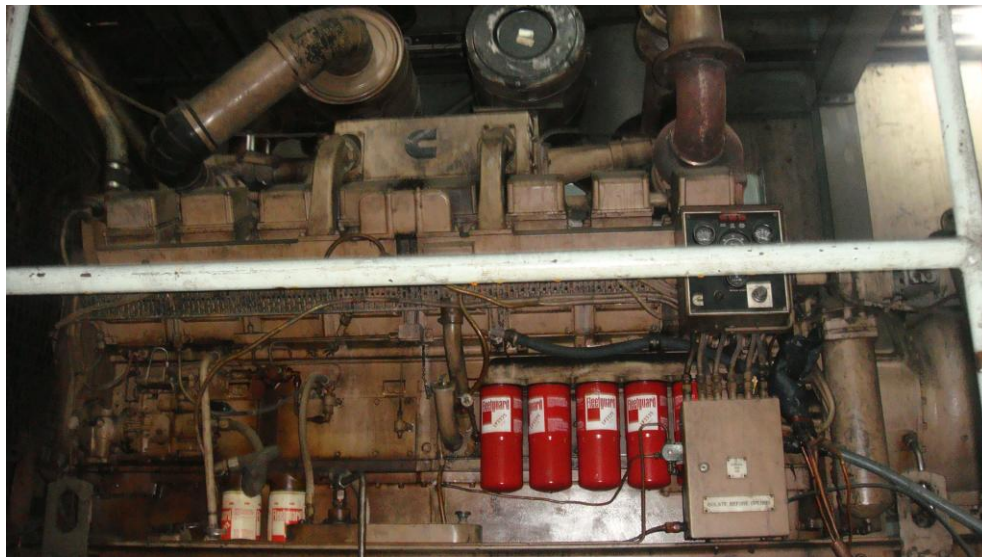
Figure 3.4 Diesel engine of combine cycle power plant.
