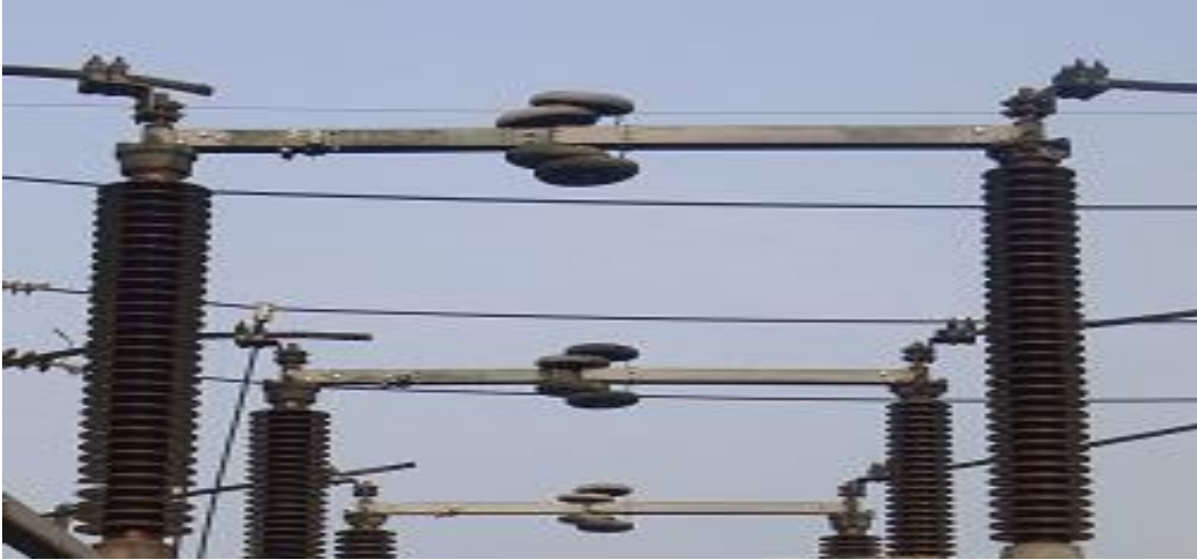
Figure 4.7: Isolators used in APSCL [Source: Author]
