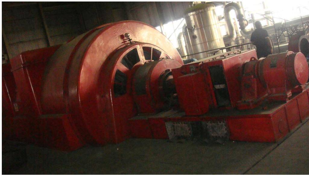
Figure 5.1: Generator in APSCL. [Source: Author]
