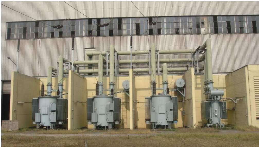
Figure 5.9: Duct use in APSCL. [Source: Author]
