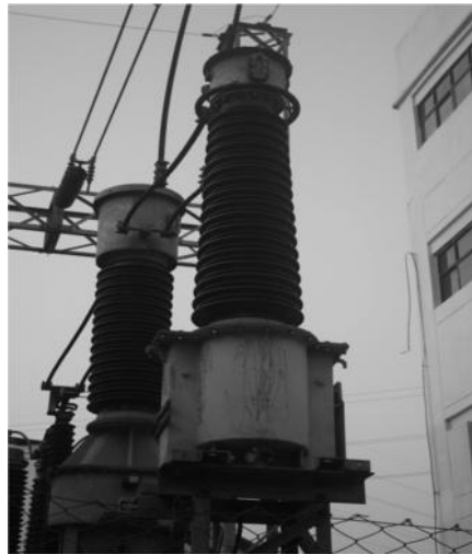
Figure 3.4: Potential Transformer at the EGCB power plant [2]
