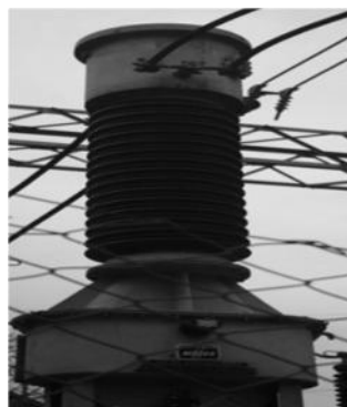
Figure 3.3: Current Transformer at the EGCB power plant [2]
