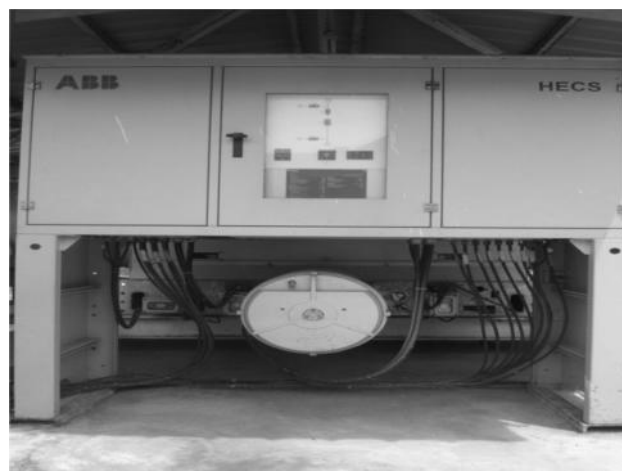
Figure 3.10: SF 6 Circuit Breaker used at the EGCB Power Plant [2]
