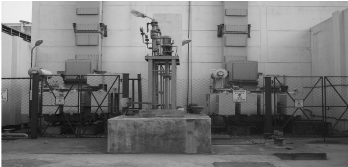
Figure 3.6: Station Auxiliary Transformer used at the EGCB Power Plant [2]
