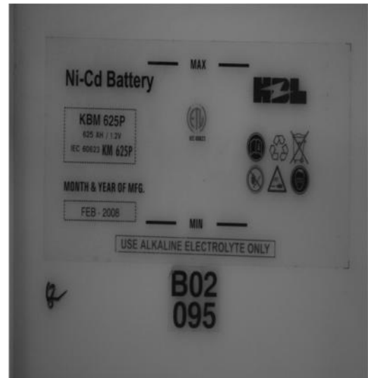
Figure 3.8: Ni-Cd Battery used for the DC Auxiliary System at the EGCB Power Plant [2]
