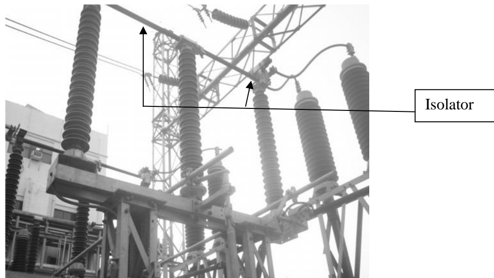
Figure 5.4: Isolators used at EGCB Power Plant [2]
