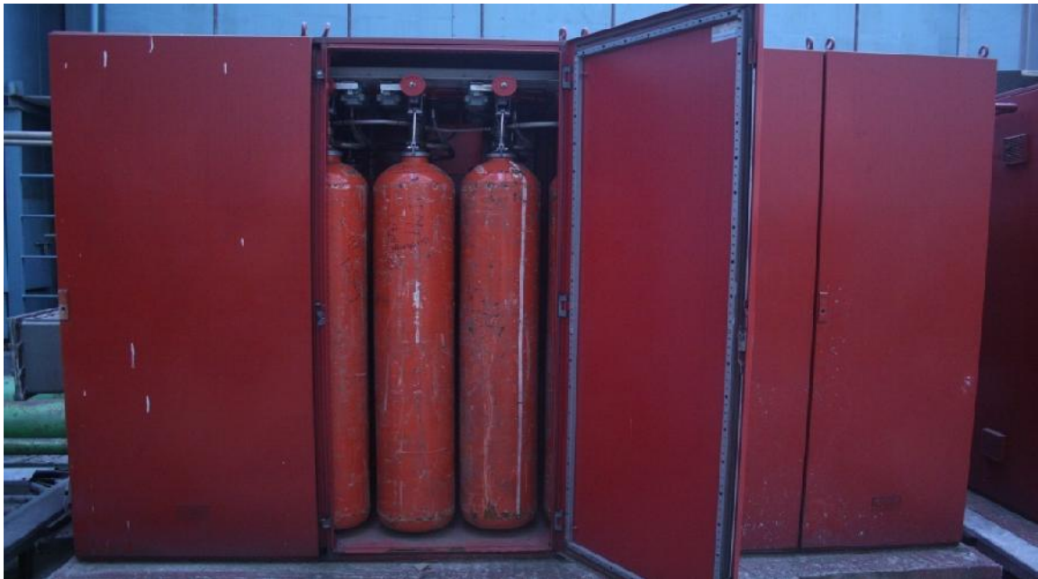
Figure 5.5: CO 2 cylinders for fire safety at the EGCB power plant [2]
