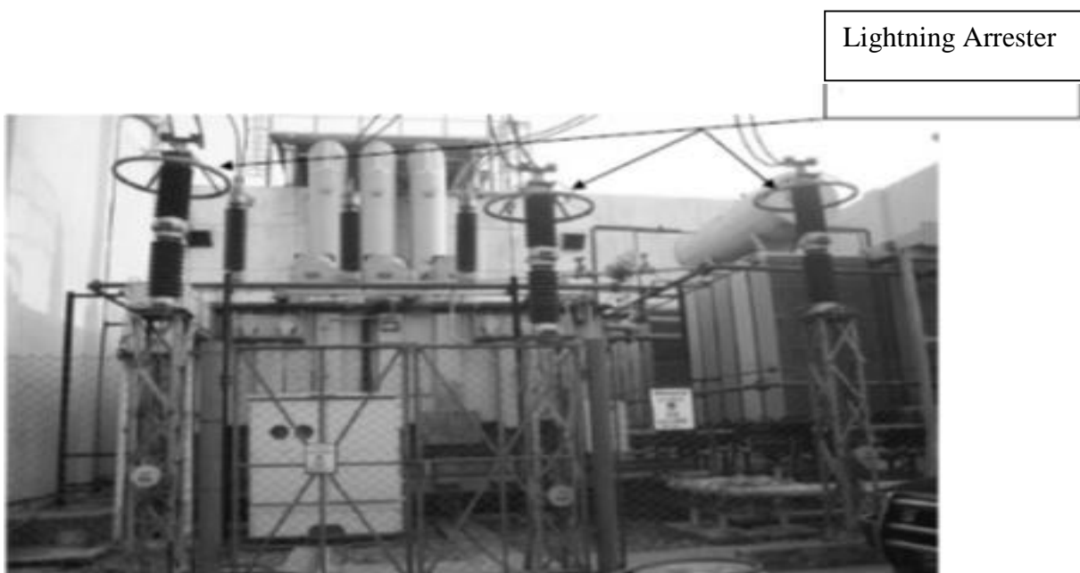
Figure 5.3: Lightning Arrester used at the EGCB Power Plant [2]
