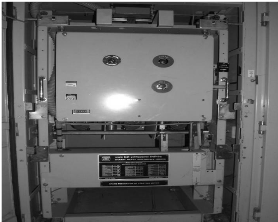
Figure 3.11: Vacuum Circuit Breaker used at the EGCB Power Plant [2]
