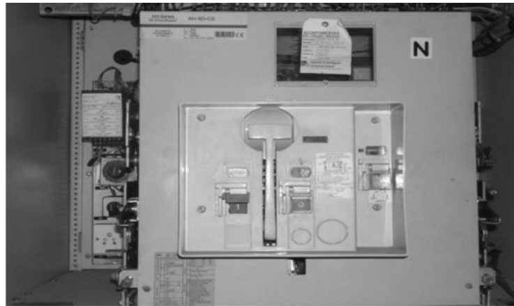
Figure 3.9: Air Circuit Breaker used at the EGCB Power Plant [2]
