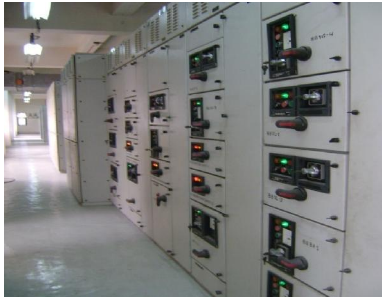
Figure 6.2: One Side of the Manual Control Room at EGCB Power Plant [3]
