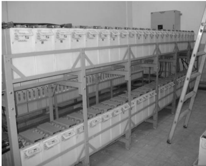
Figure 3.7: The DC Auxiliary System storage facility at the EGCB Power Plant [2]
