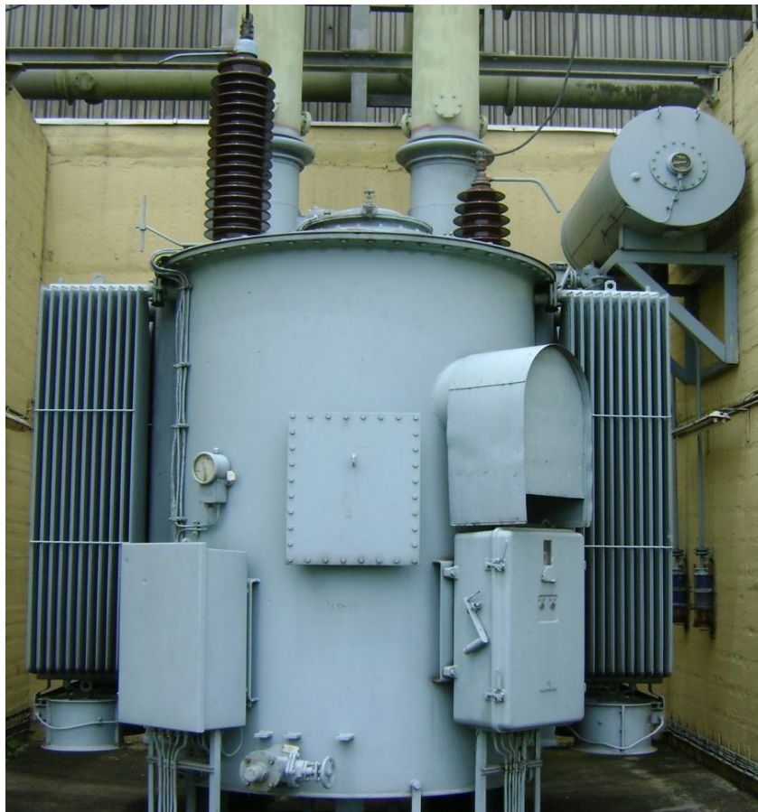
Figure 3.1: Single Phase Transformer at APSCL [7].
