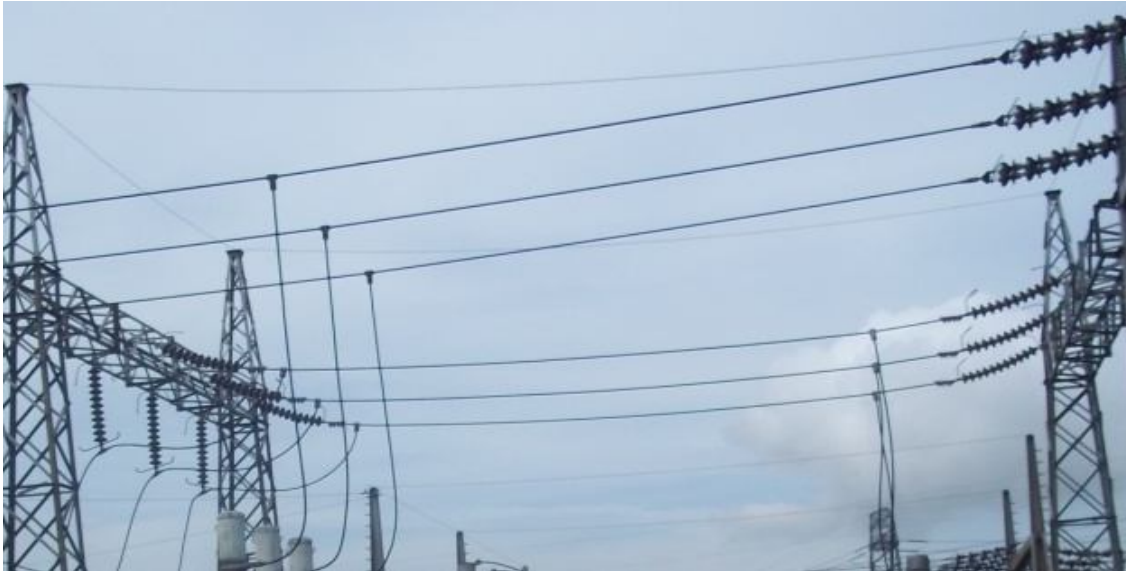
Figure 5.2: Over Voltage Protection at APSCL [7].
