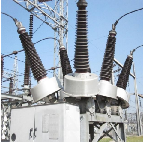
Figure 5.9: SF6 Circuit Breaker at APSCL [7].
