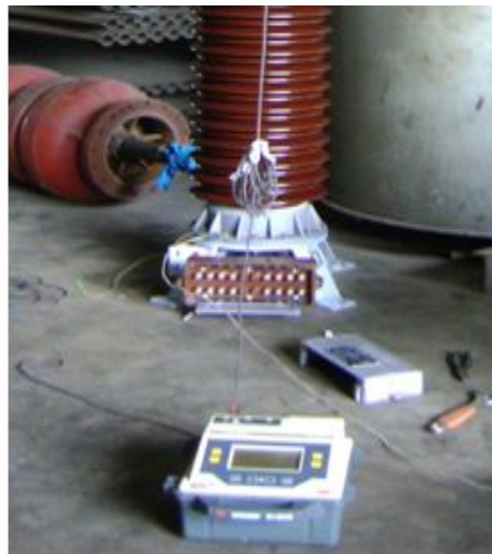
Figure 4.3: Megger Test Machine at APSCCL [7].
