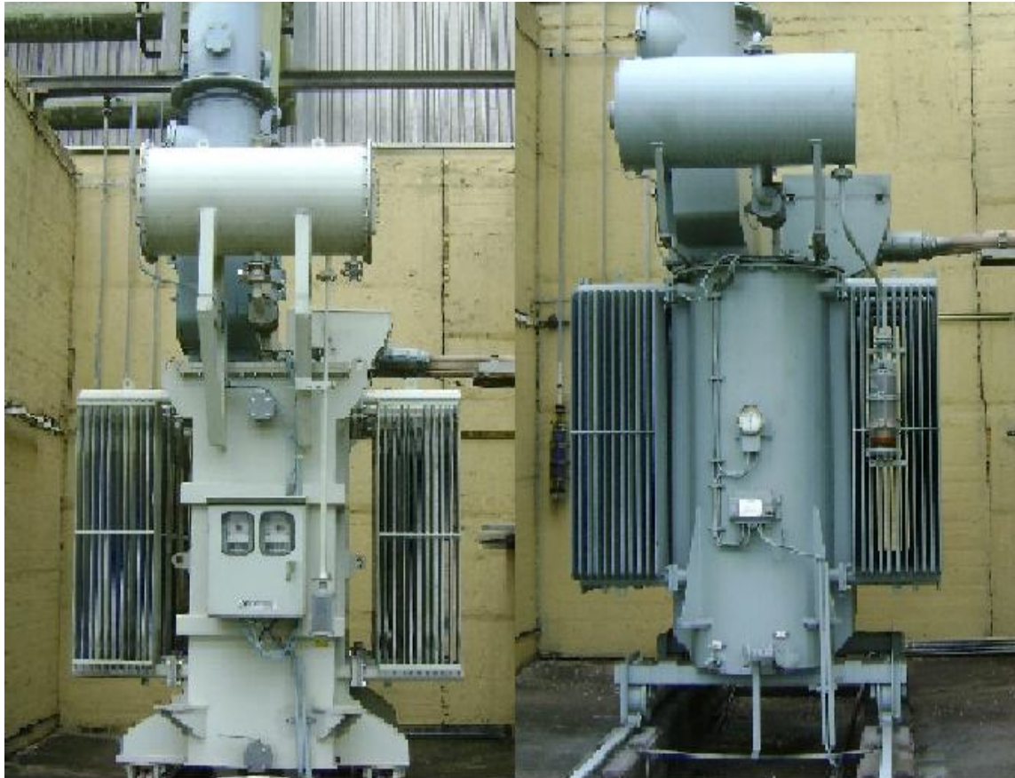
Figure 3.3: Auxiliary Transformers at APSCL [7].
