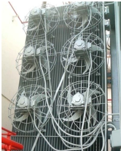
Figure 3.5: Cooling Fans of Transformer at APSCL [7].
