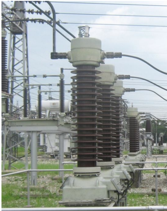
Figure 4.5: 132 kV Voltage Level PT at APSCL [7].
