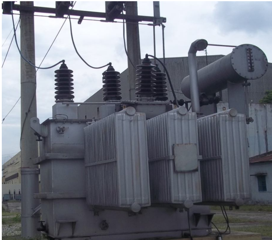
Figure 3.2: Earthing Transformer at APSCL [7].
