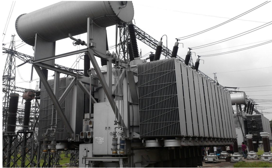
Figure 3.4: Coupling Transformer between 132 kV and 230 kV Buses [7].
