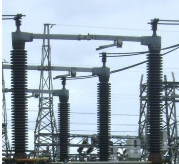
Figure 5.1: Isolator at APSCL [7].
