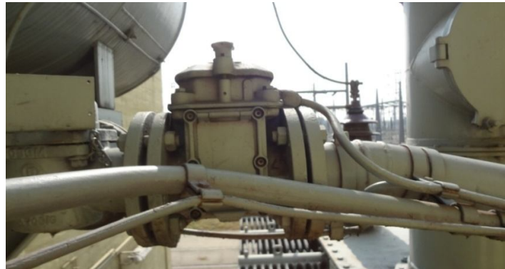
Figure 3.6: Buchholz Relay of Transformer [7].
