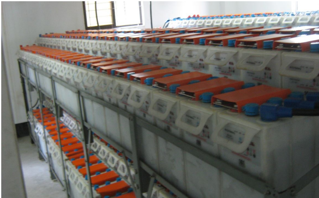
Figure 5.11: Battery Room of Substation at APSCL [7].
