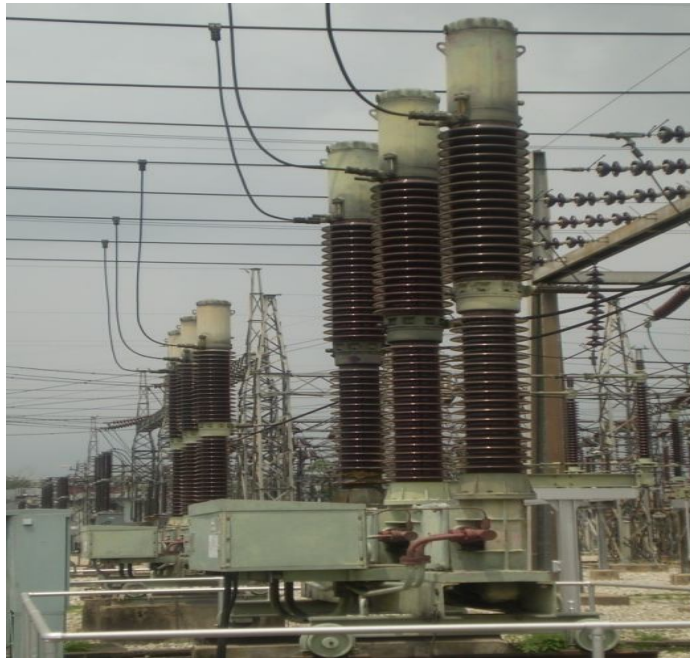
Figure 5.8: Oil Circuit Breaker at APSCL [7].
