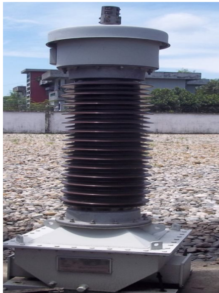
Figure 4.6: 230 kV Voltage level PT Reduces Line Voltage [7].
