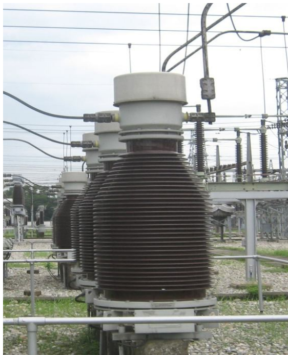
Figure 4.2: 132 kV Voltage Level CT at APSCL [7].
