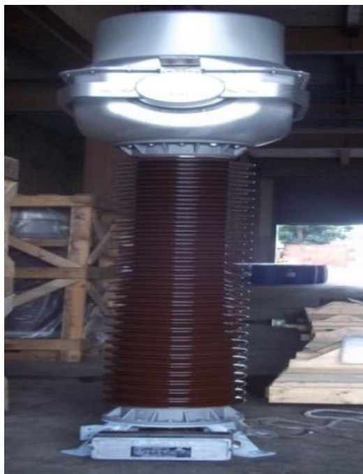
Figure 4.1: 230 kV Voltage Level CT at APSCCL [7].
