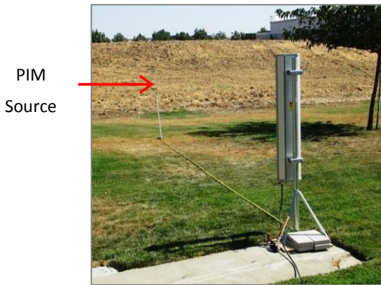
Figure 5.3 PIM source 30 ft (9.1m) in front of an antenna
