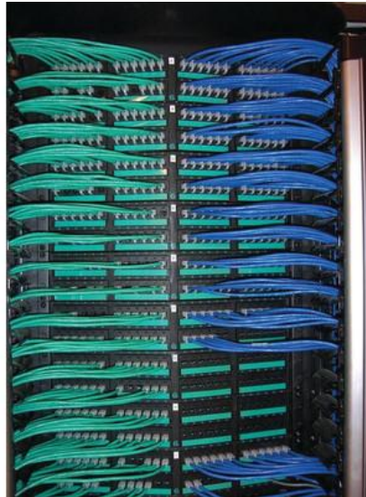
Figure: Structured Cabling
