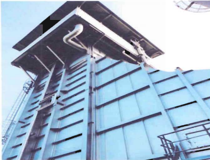
Figure 4.9: Boiler of MPS
