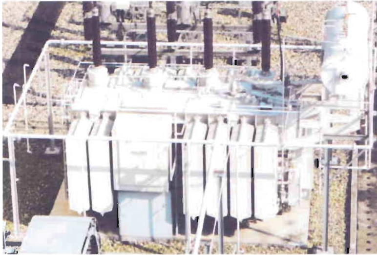
Figure 3.4: A power transformer 11 kV to 132 kV
