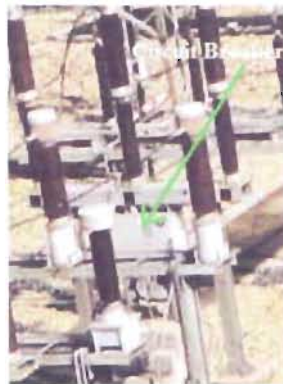
Figure 3.7: SF6 Circuit Breaker, 6.0 bar pressure by ABB (Sweden)
