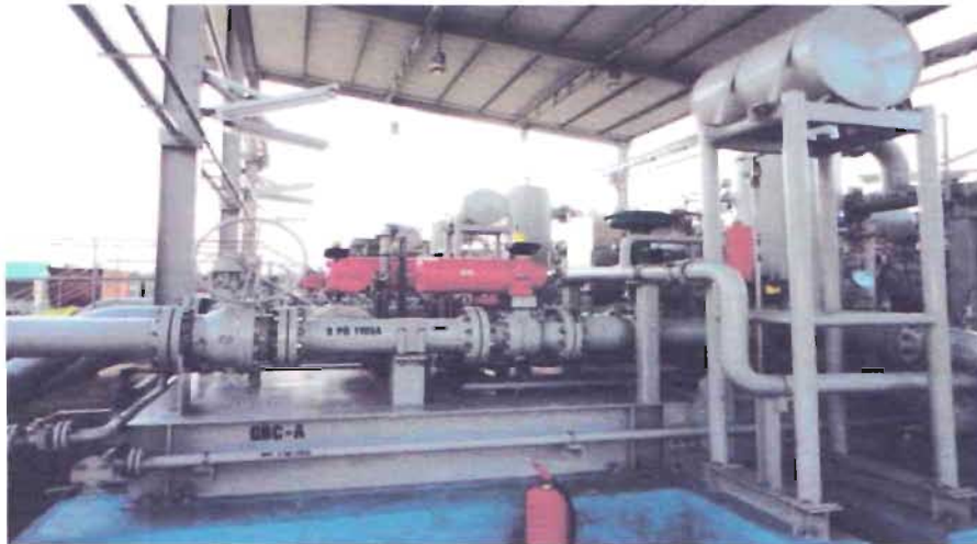
Figure 4.6: Gas Booster of MPS
