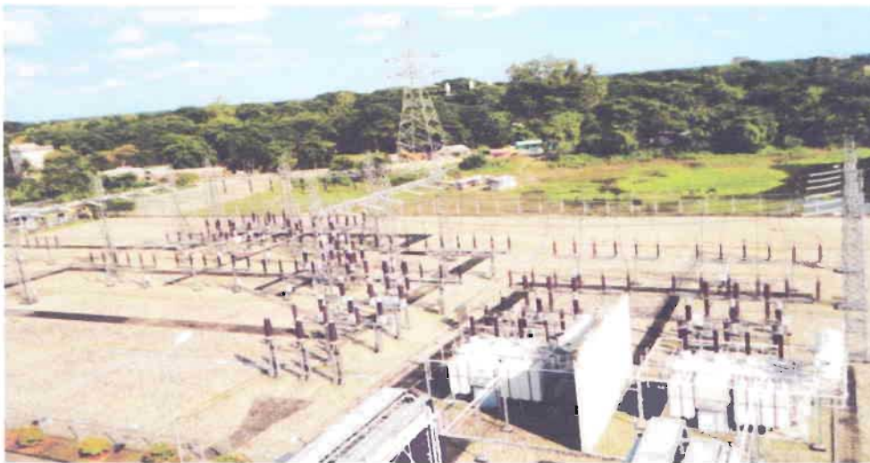
Figure 3.1: A 11/132kV substation in Mymensingh power station (MPS)
