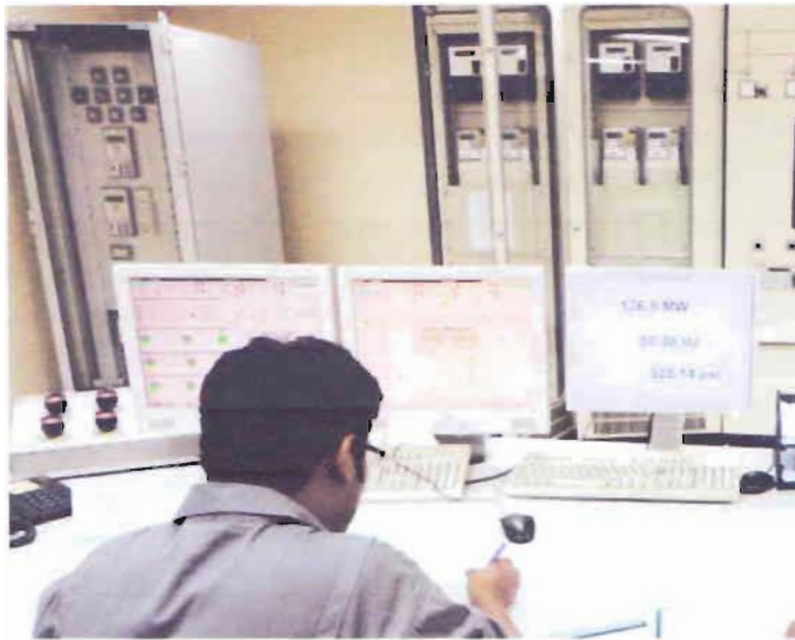
Figure 3.12: Monitoring generation from Central Control Room in MPS
