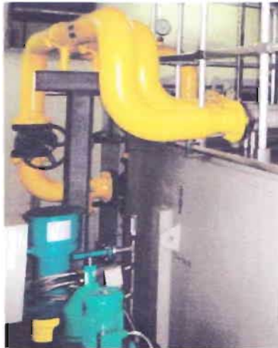
Figure 4.10: Lube Oil Pump
