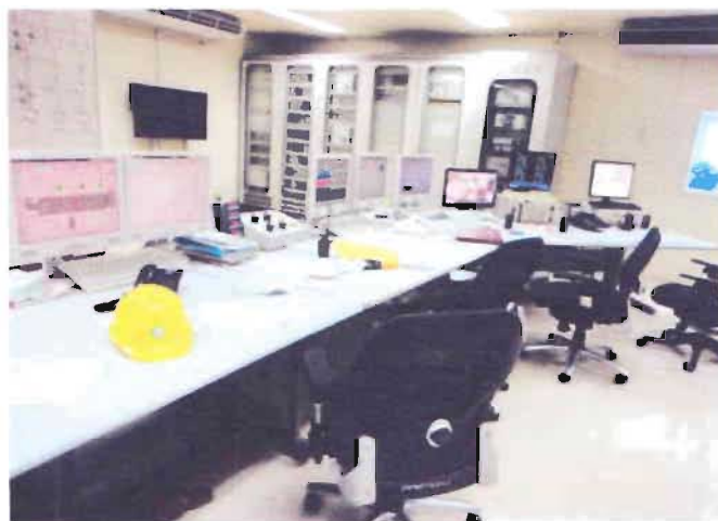
Figure 6.1: Central Control Room of MPS
