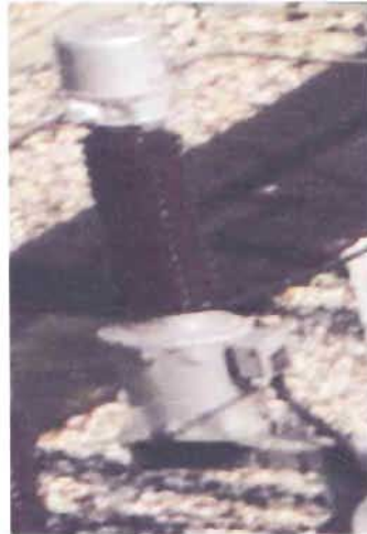
Figure 3.5: Current Transformer by ABB (Sweden) used in MPS's substation
