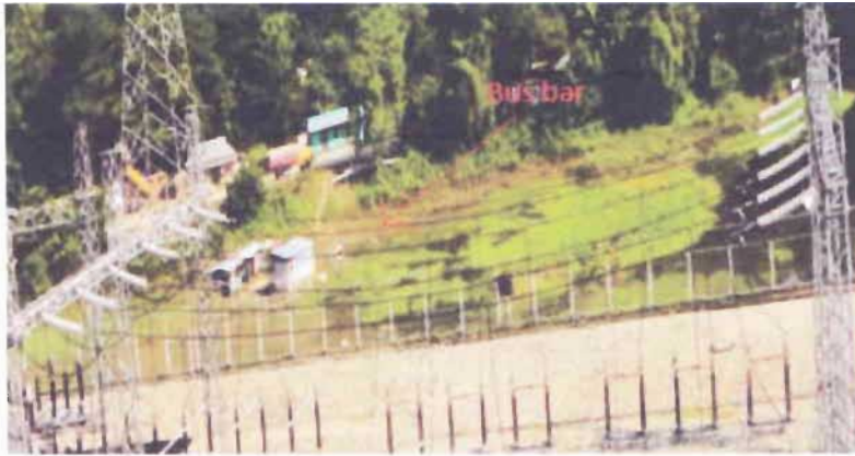
Figure 3.9: A double Bus bar is used in Substation in Mymensingh power plant
