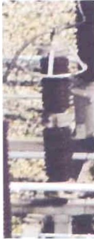
Figure 3.8: Lightning Arrester in the substation of MPS
