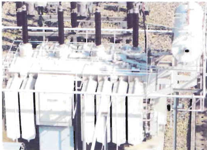
Figure 2.9: Transformer of MPS
