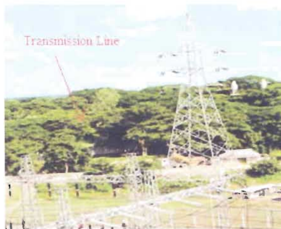
Figure 3.10: Transmission Lines in MPS
