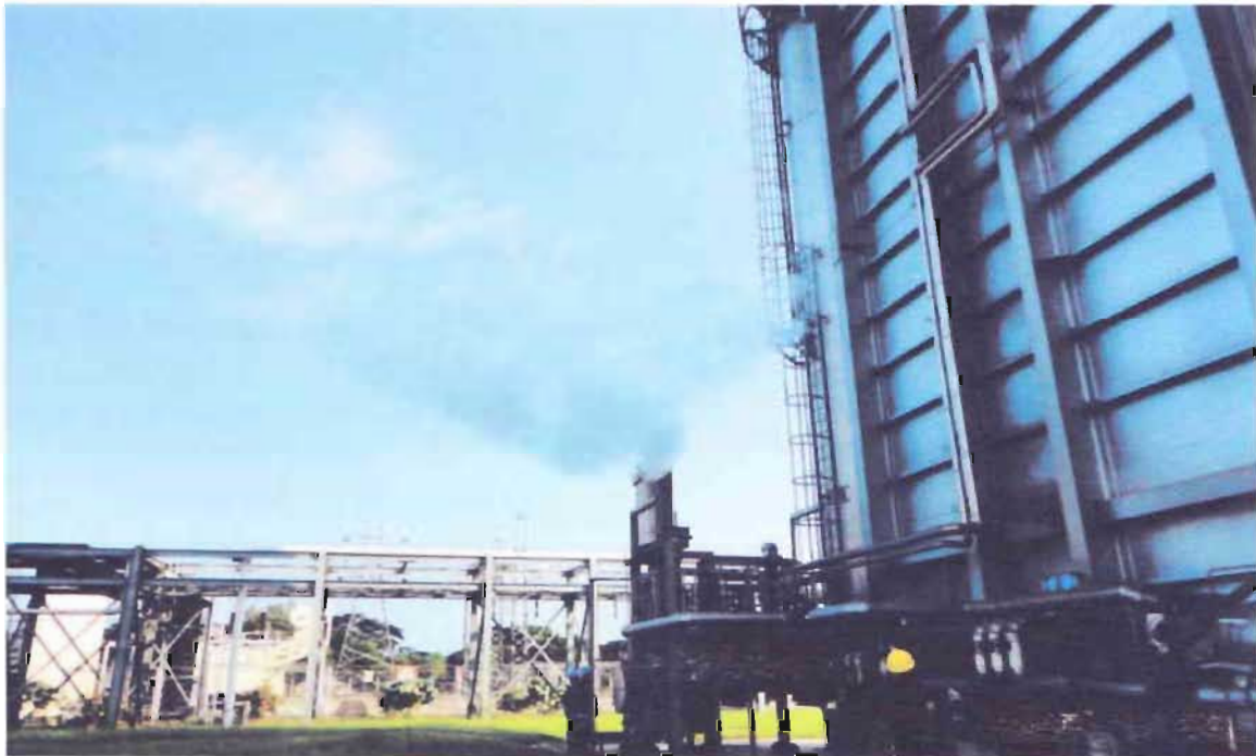
Figure 4.7: Steam power station of MPS
