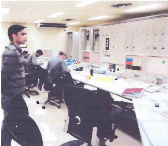
Figure 3.11: Control room of substation in MPS
