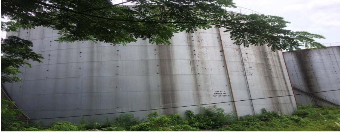
Fig 4.9: Storage Tank for HFO.
