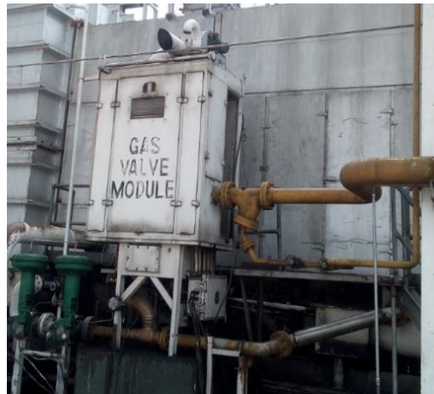
Fig 3.13: Gas valve module
