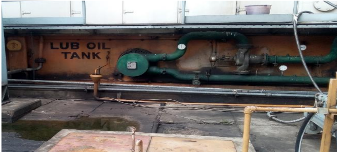
Fig 3.10: Lubricating oil tank of Baghabari gas turbine power plant
