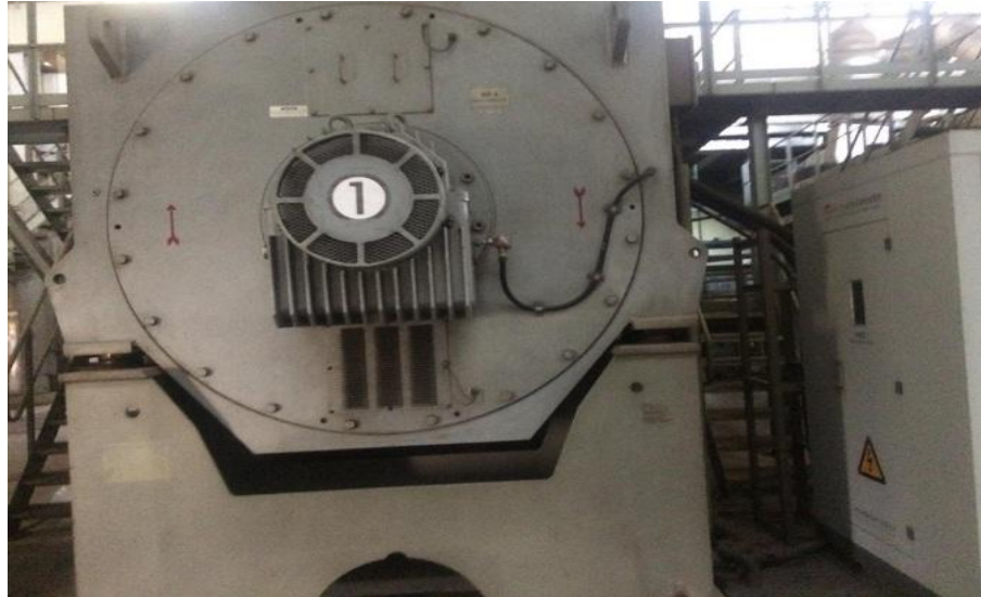
Fig 2.5: Engines are coupled with the Generators at Katakhalipower plant
