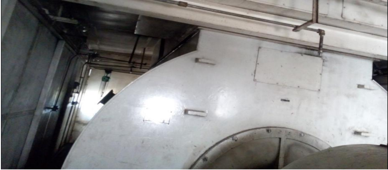
Fig 3.6: Generator of Baghabari gas turbine power plant
