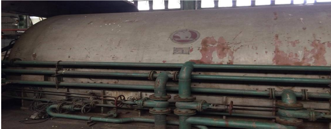
Fig 4.2: A view of 110 Generator at Khulna power plant
