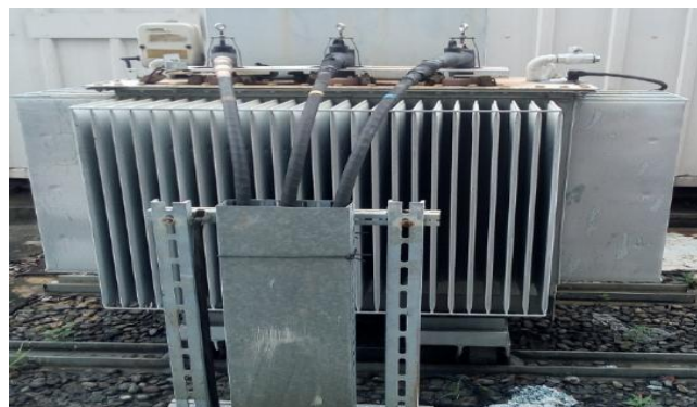
Fig 3.8: Auxiliary Transformer of Baghabari gas turbine power plant
