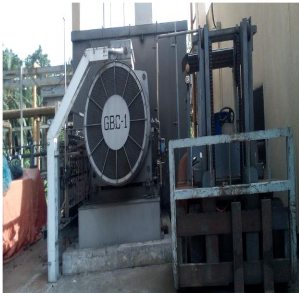
Fig 3.12: Gas booster units
