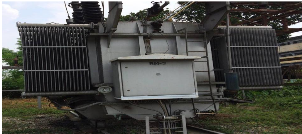
Fig 4.11: Unit Transformer of Khulna Power Plant
