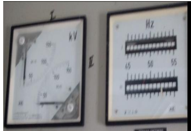
Fig 3.17: Voltmeter and frequency meter
