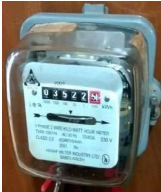
Fig 7.1: Single Phase Energy Meter (Analog)
