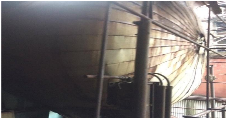
Fig 4.5: A view of Boiler Drum at Khulna power plant
