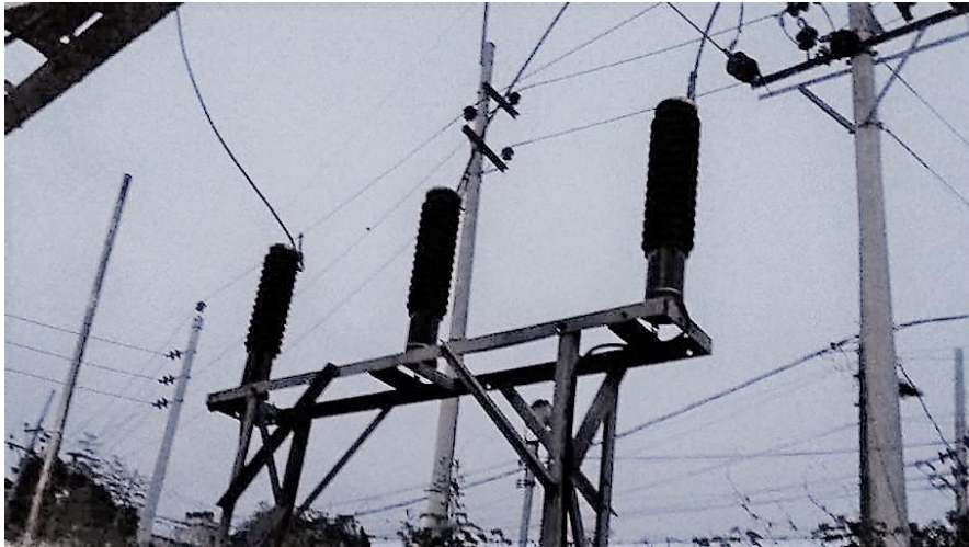
Fig 6.3: Lightning arrester of Horogram substation
