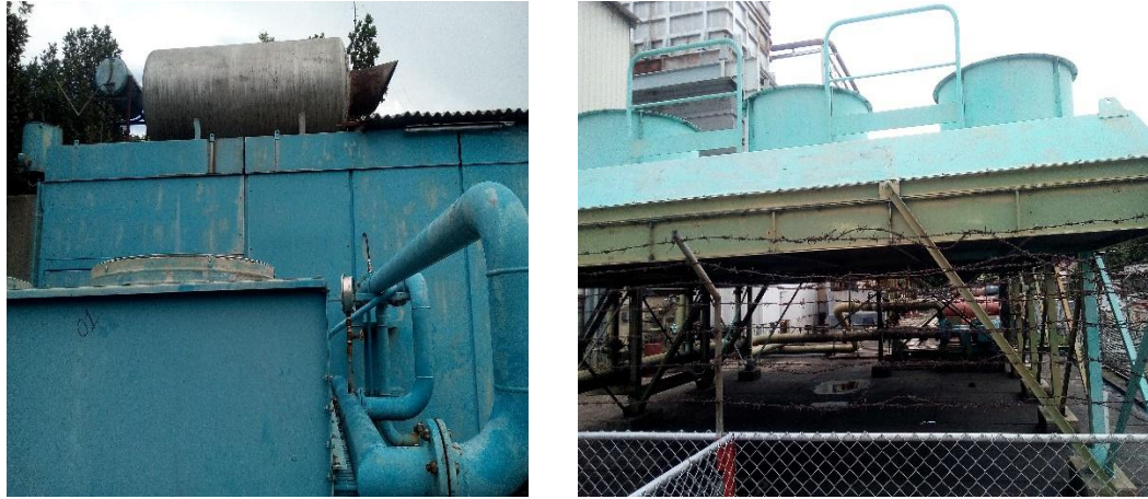
Fig 3.14: Water treatment plant of Baghabari gas turbine power plant
