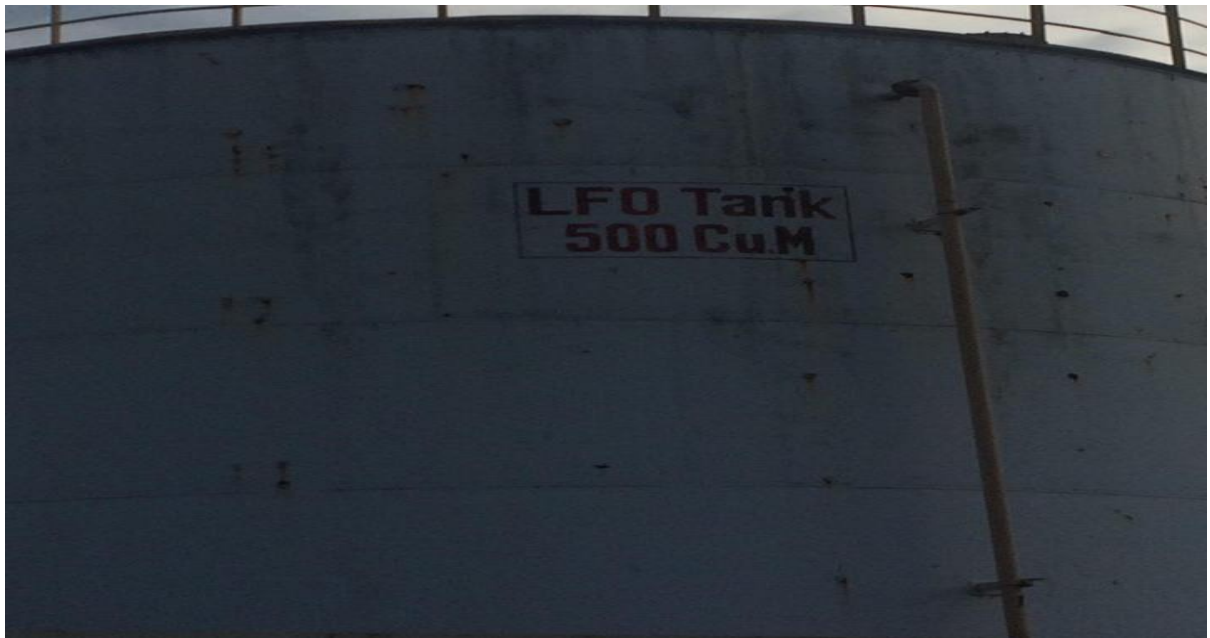
Fig 2.2: LFO tank at Katakali peaking power plant
