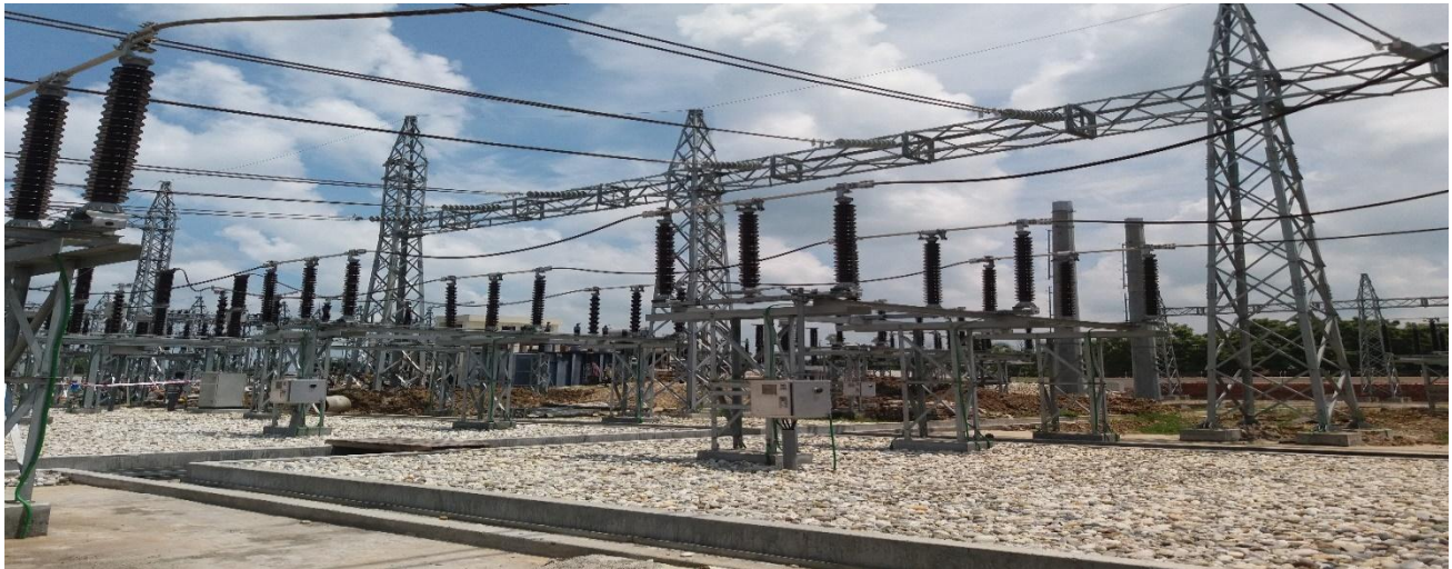
Fig 5.2: double line bus bar at Amnura substation
