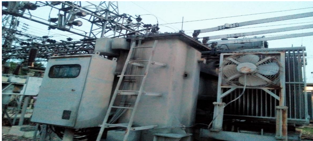
Fig 6.1: Step down transformer
