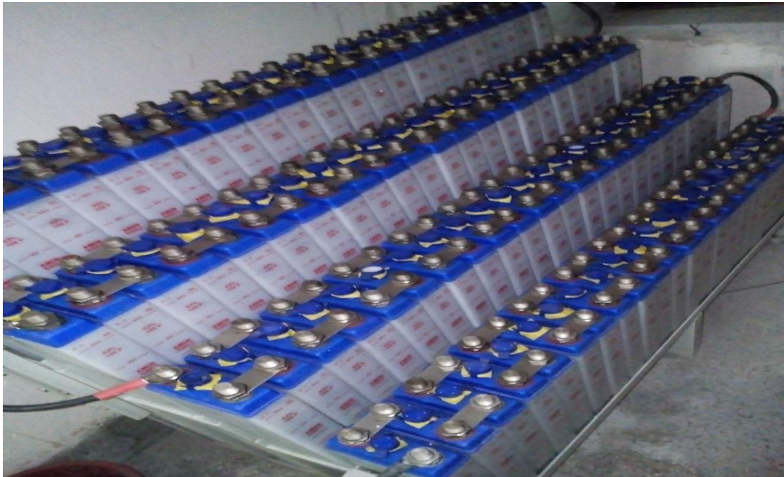
Fig 6.2: Battery Bank of Horogram substation
