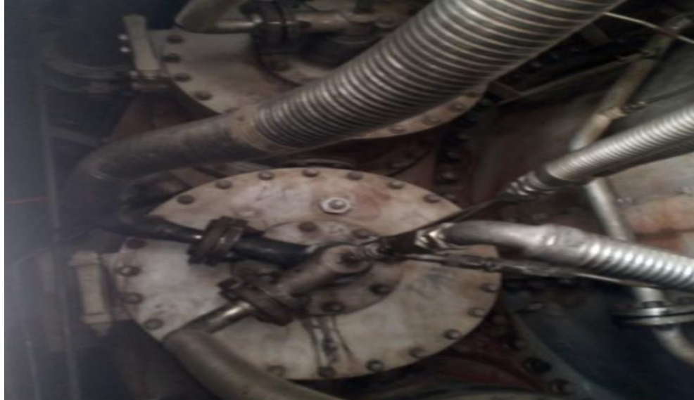
Fig 3.4: Burner of combustion chamber
