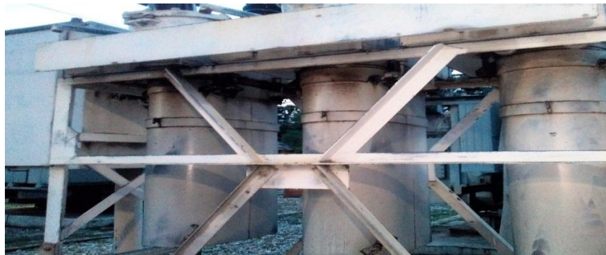
Fig 6.5: Oil circuit breaker of Horogram substation
