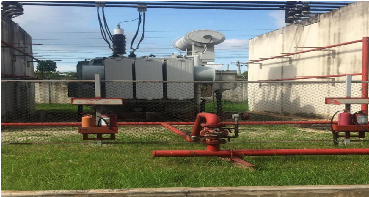
Fig 2.3: 11/132KV Transformer at Katakali power plant
