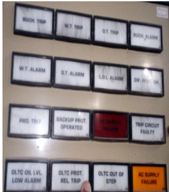
Fig 6.8: Alarming system of control room
