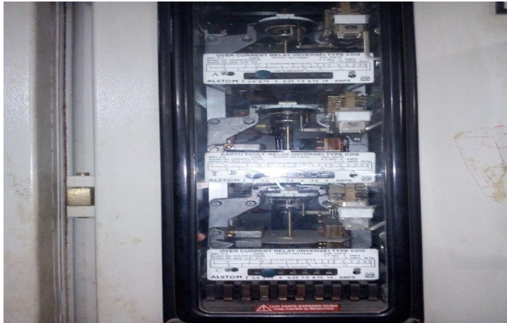
Fig 6.6: Overcurrent relay of Horogram substation
