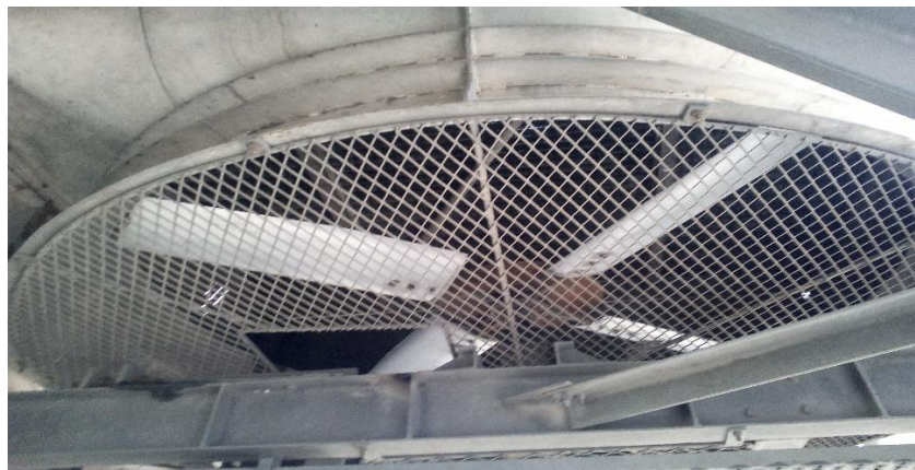
Fig 3.15: Air cooling fan of Baghabari gas turbine power plant
