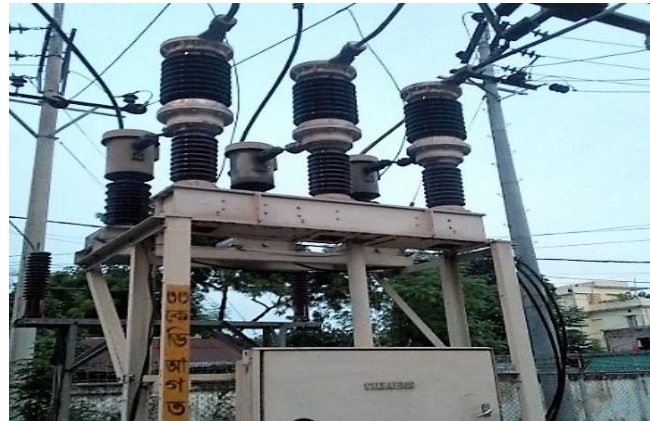
Fig 6.4: SF 6 circuit breaker of Horogram substation
