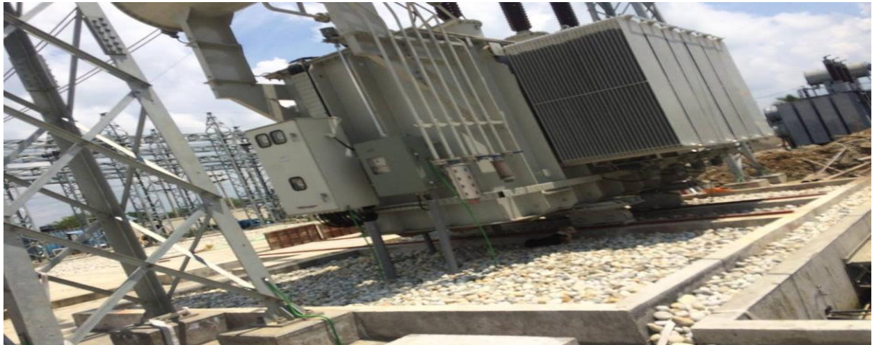
Fig 5.1: 132/33 KV transformer of Amnura grid substation
