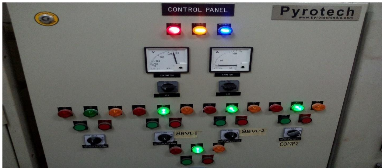
Fig 3.9: Control panel of Baghabari gas turbine power plant
